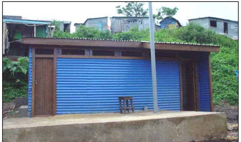
Picture 2 Installed gender separated public toilet at the Kerebe-Landing Site
